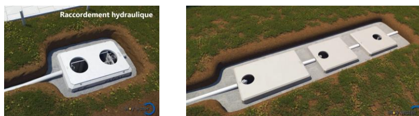
Fig-23: Hydraulic Connection
