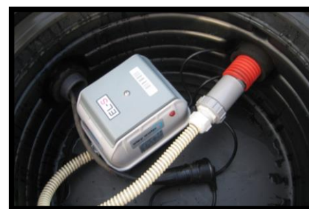
Figure-29: Electrical Connection in utility chamber
